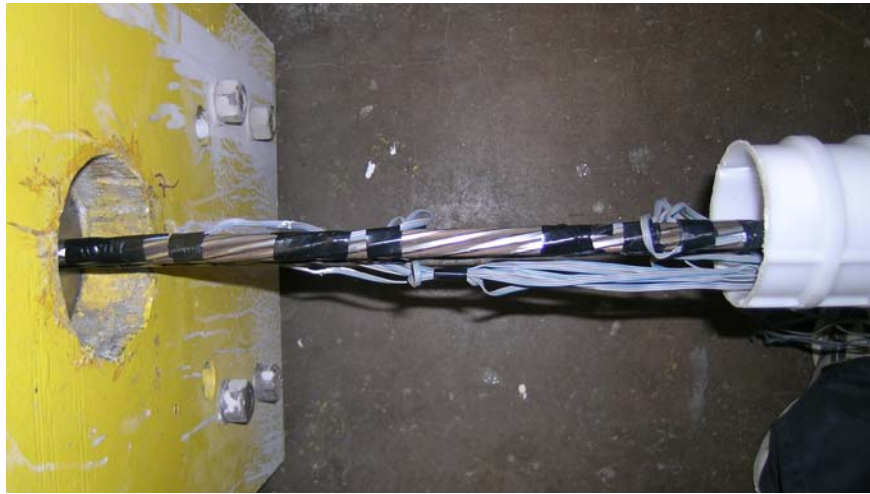
Figure 3-10 Strain gages on strands at north end with duct shifted to the side
