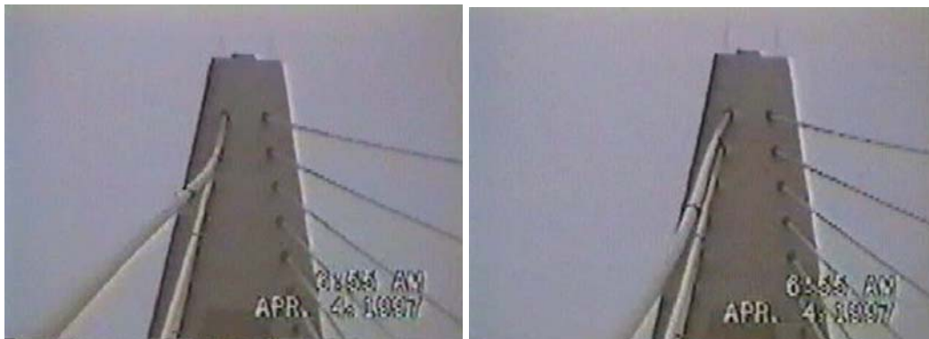
Figure 1-6 Observed large-amplitude vibrations of stay cables on Fred Hartman Bridge (TxDOT, 1997)
