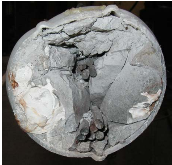
Figure 6-9 Photograph of condition of specimen after fracture at north end of Specimen 1
