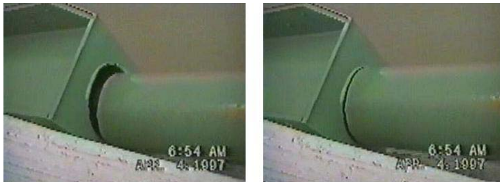
Figure 1-7 Broken guide pipe to anchorage box connections (TxDOT, 1997)
